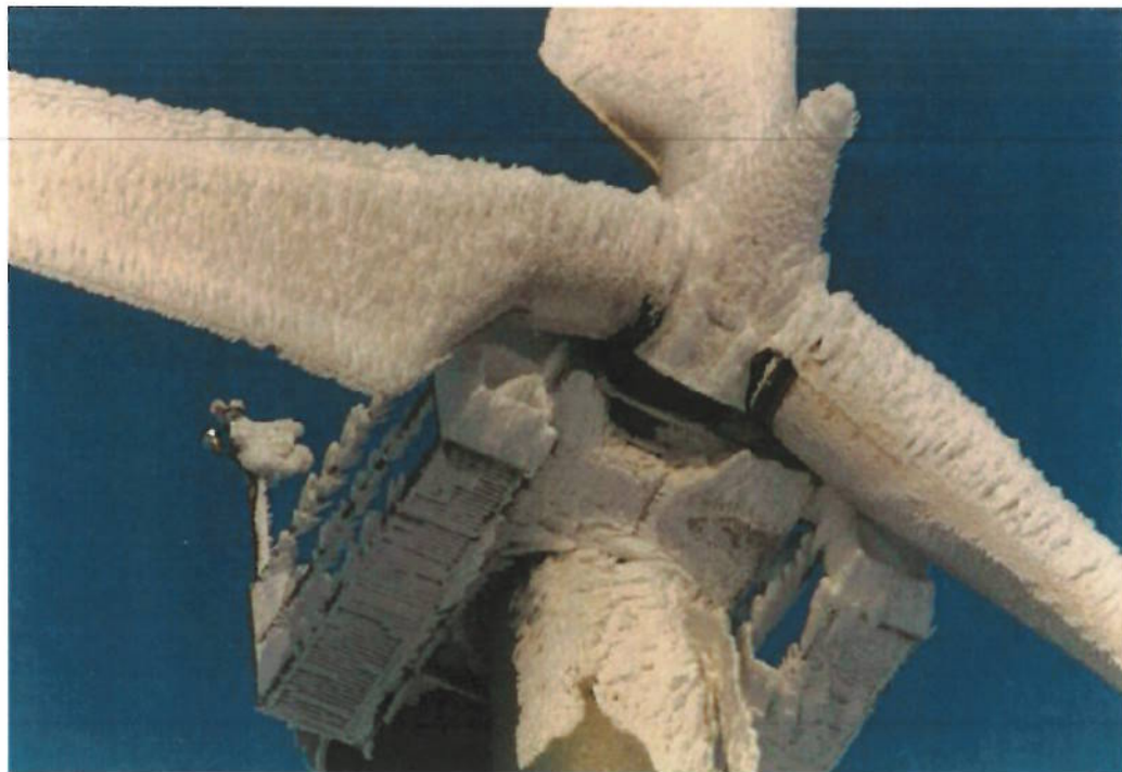
Photograph 4: wedge shaped ice builds up on the blades when running through icing events – leading edge heaters not working
