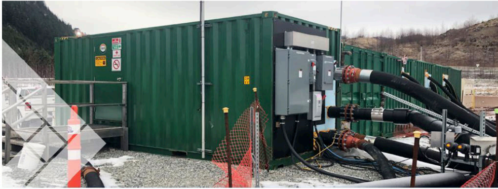
Figure 4-5: Chitosan Enhanced Sand Filtration (CESF) Management Systems (Figure Courtesy of SECURE)
